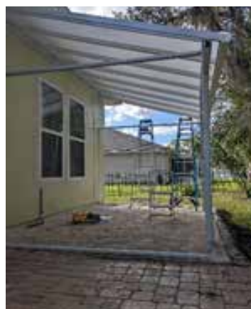
The first step was installing pavers for the foundation of the structure
