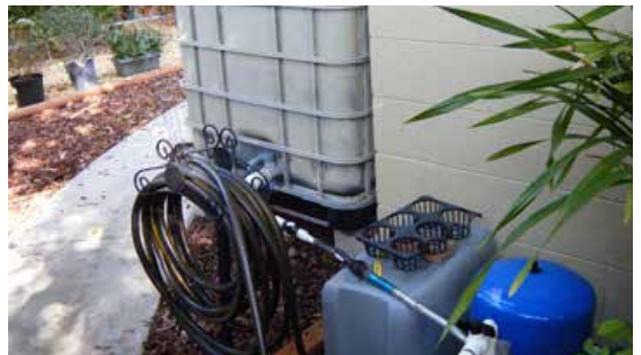
Rainwater collection & pumping system
